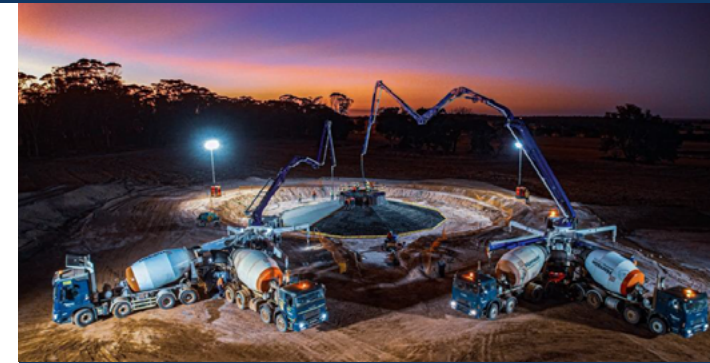
Tier 1 miner, Nickel. Wind Farm Stage 1, WA 18x 4.2MW WTG Foundations, Pads, Access Roads Design for Construction Contractor, 2022. Value added: optimised size of foundations and segmental reinforcement.
